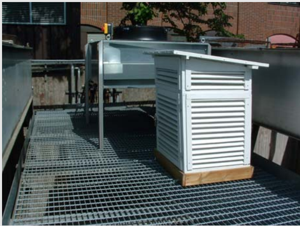
Dry cooler and Stevenson screen for sensors.
