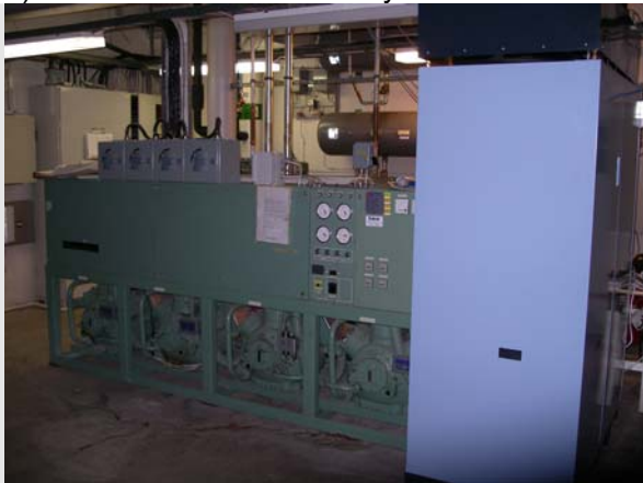
Main compression chiller (left) and TDC (right).
