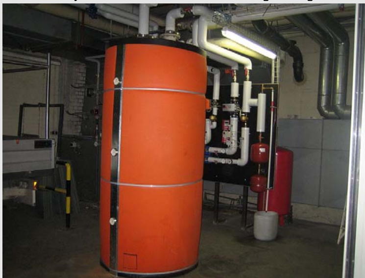
Hydraulic installation with mixing storage
